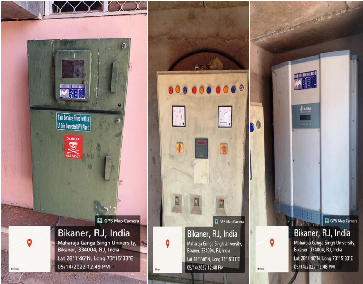
100kwp Grid connected SPV Power
